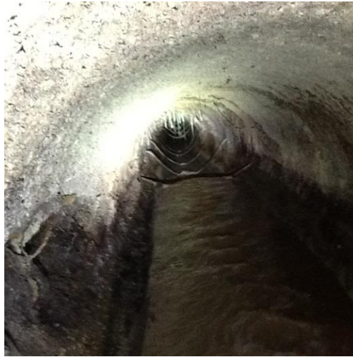
Milliscreen Trunk Sewer showing severe concrete corrosion
