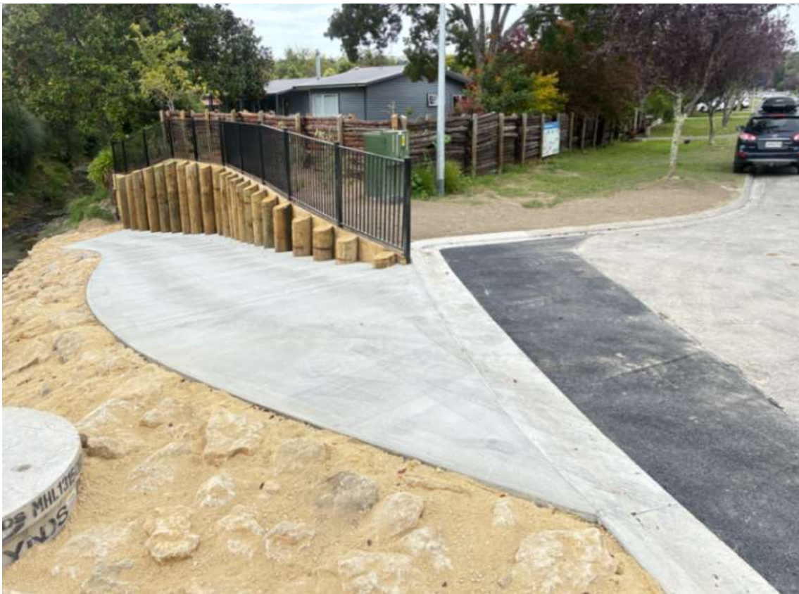
Figure 2: Completion of Stage - Sep Portion 2 Plassey Access and Bank Remediation at 7 March 2026
