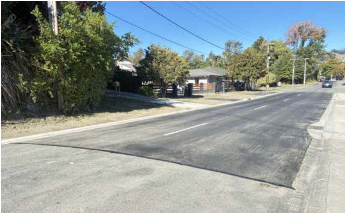
Figure 3: Stage 1 - Seperable Portion 3 - SW Pipe Upgrades and Road Recontouring Complete at 13 Apr 2026
