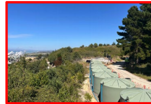
Whirinaki temporary tanks and pad for new reservoir above
